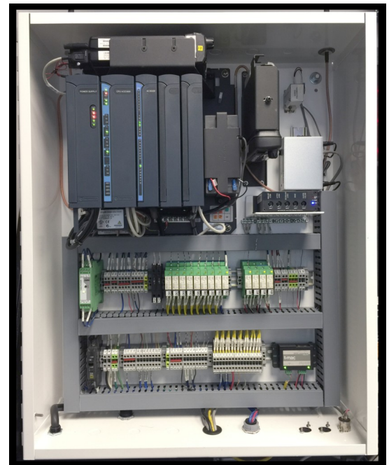
MACH Alert Station Controller (SC) (Typically one per Fire Station)
